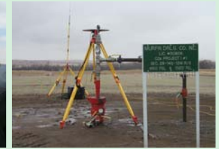
Figure 7. GPS base station at CO 2 injector.
