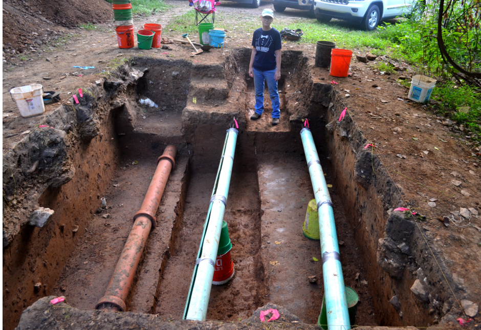
Figure 9. Electrical cable lines (right), sewer line (left), and water line (upper left) in Block A (view to east).
