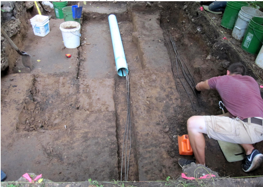
Figure 8. Electrical cable lines in Trenches 1 and 3 in central and southern portions of Block A (view to west).
