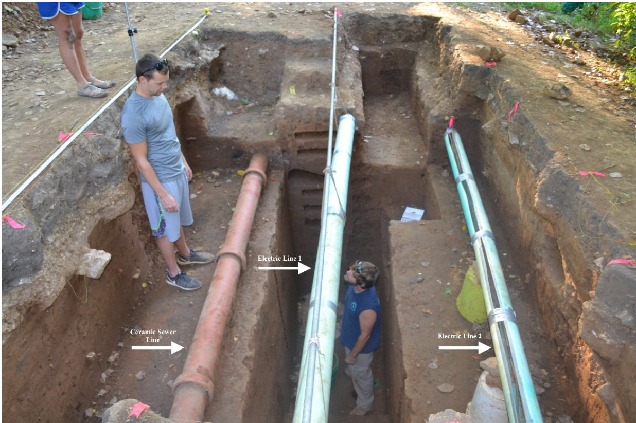
Figure 6. Photograph of electric lines and ceramic sewer line. PVC pipe was placed around electric lines to prevent accidental damage during excavation and backfilling by the Odyssey team. View to the east.
