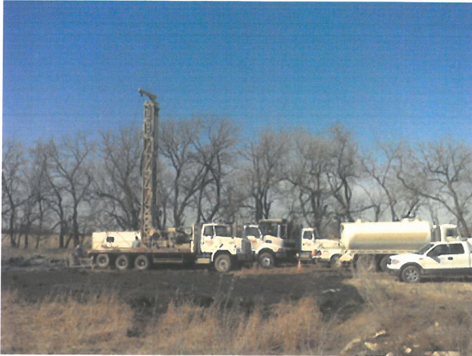
STOP #1—Drilling Rig: McPherson Drilling. PostRock Energy will be drilling the Taylor, James P. 7-1. Located in NE/4, NW/4, Sec. 7, T.35S.R., 18E., Labette County.
