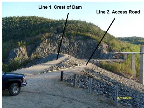
Figure 2. View to the south from the dam crest. Seismic data were acquired at the crest of the dam and along the access road.
