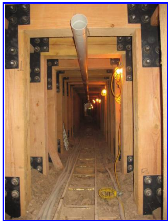
Figure 2. Picture of the inside of the test tunnel displaying wood shoring, rail tracks, ventilation pipe, and electric lighting.
